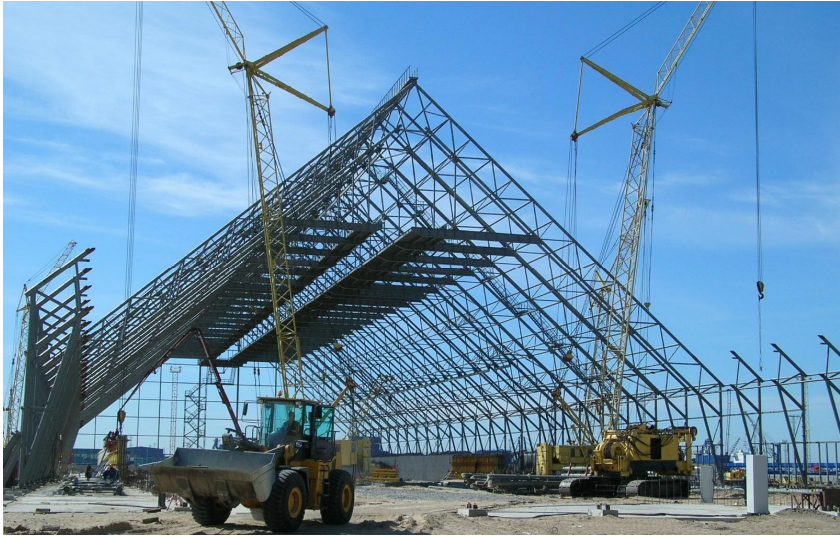
Fig. 3.1. Assembling process on job site (Photo has been provided by V. Shymanovsky Ukrainian Research and Design Institute of Steel Construction)
