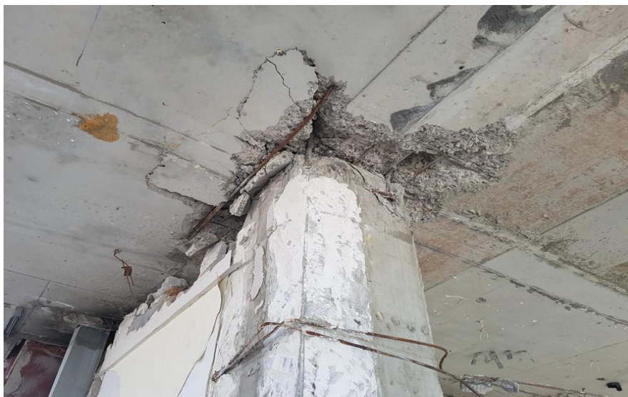
Fig. 3. Concrete fractures of columns at punching zone of floor slabs
