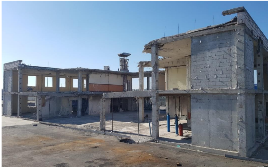
Fig. 2. General view of the partially collapsed building
