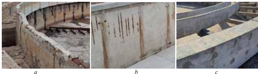
Fig. 1. – Condition of structures at wastewater treatment facilities №2 (Kharkiv) a – tray of settling tank; b – aeration tank walls; c – restored of settling tank structures
