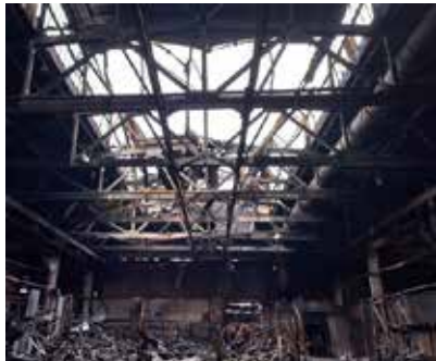
Fig. 1 - Collapse of the skylight structure
