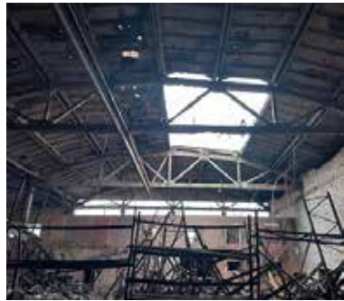
Fig. 2 - Destruction and damage of the roof slabs due to dynamic impact with subsequent fire development
