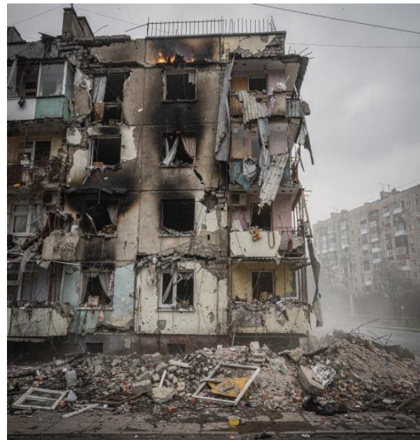
Fig. 2. Façade destruction in residential building, Kyiv (example of moderate to severe damage classification)
